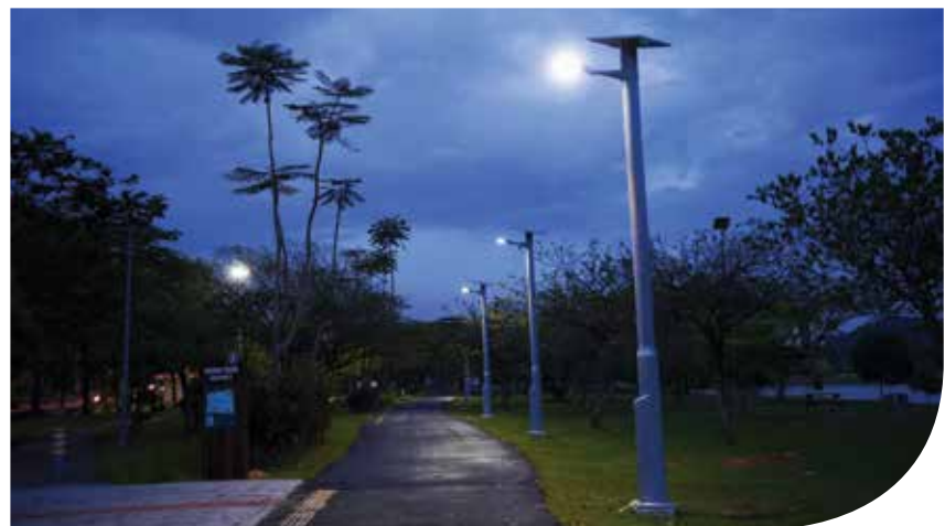
SIRIM solar powered streetlights with built-in lithium-ion batteries and composite poles installed at Taman Tasik, Section 7, Shah Alam
