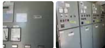
OLU UNIT AT SUBSTATION NO. 6 - PROJECT COMPLETED ON 26 DECEMBER 2019
