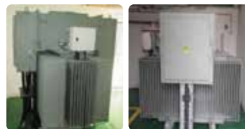
TRANSFORMER AT SUBSTATION NO. 2 - PROJECT COMPLETED ON 28 SEPTEMBER 2019
