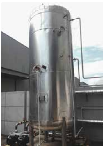
THERMAL ENERGY STORAGE
