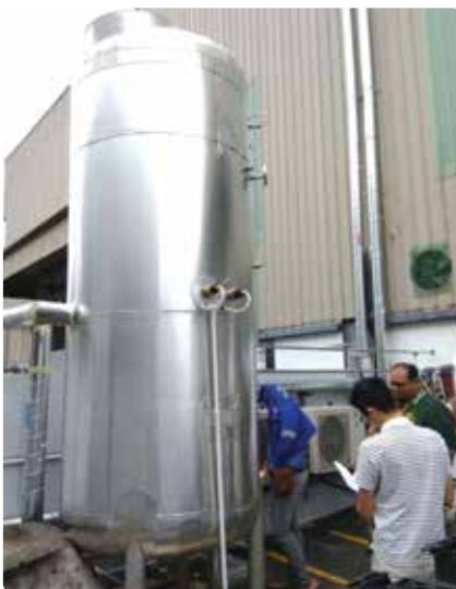
4000L HEATED WATER TANK
