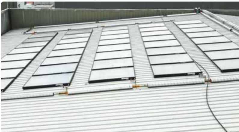
SOLAR COLLECTOR ON ROOF TOP
