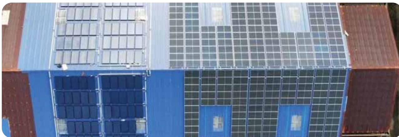
Solar Thermal and Solar PV installed on a rooftop
