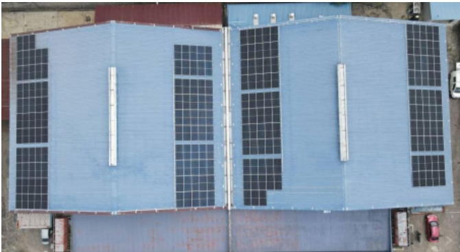
Solar power system at SIRIM Jalan Lada Sulah
