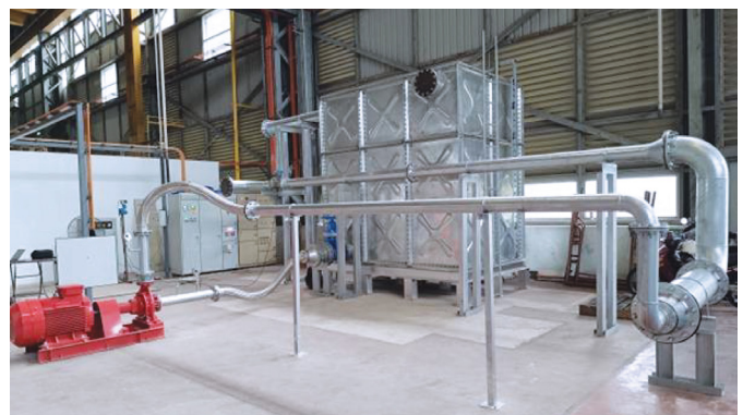
Fire Pump Testing Facilities for SIRIM QAS International Sdn. Bhd.
