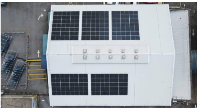
Solar power system at SIRIM Jalan Pahat
